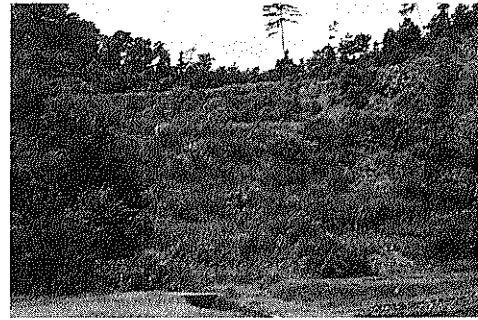
Photo 12 圃場面勾配の修正工事3年後に安定した法面 (Fig.11の圃場) Stable slope three years after the modification work
