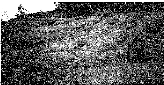
Photo 13 No.9の法面崩壊 Slope failure at No.9 slope
