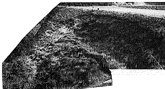
Photo 1 浅い円弧滑りによる法面崩壊 (Fig. 5のA) Slope failure by shallow slip circle
