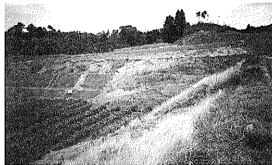
Photo 15 No.2 (遠方) 及びNo.3 (手前) の法面崩壊 Slope failure at No.2(distance) and No.3(near) slope
