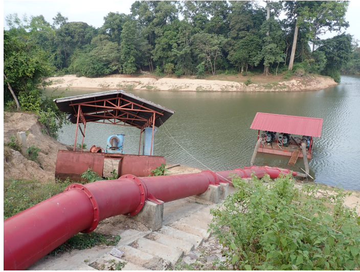
Photo 23. An irrigation facility that pumps water from a pond in the Panomsai village
