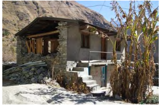
Photo 10. Damaged residence by earthquake at Goljung, Rasuwa Dist.
