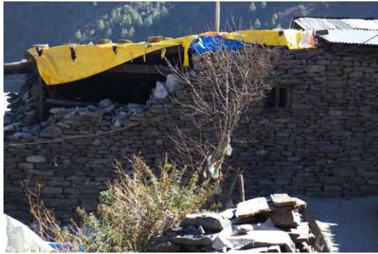
Photo 9. Damaged residence by earthquake at Goljung, Rasuwa Dist.
