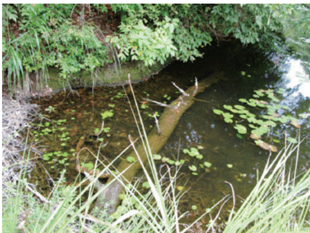
Fig.2-4 洪水吐流入口に漂着した流木 The driftwood which was cast ashore in spillway
