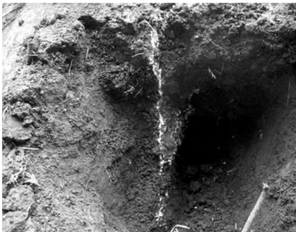
(b) Crack depth of 50 cm.
