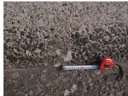
Fig. 7 農業用水路の摩耗状況 Erosion state of concrete irrigation canal
