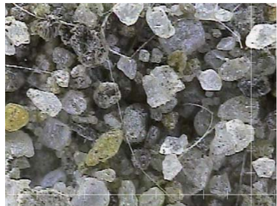
Fig. 28 補修後に摩耗された G 地区の水路状況 Eroded canal state after repair in the G district. The polymer cement paste is lost, the fine aggregate remains at the surface.
