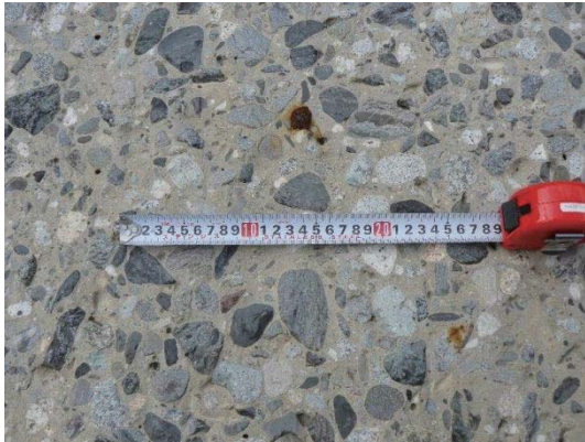
Fig. 25 F 地区（頭首工）の状況 Apron state of head works in the F district
