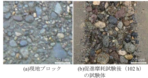
Fig. 60 摩耗状況の比較 Comparison of erosion state of surface at an actual canal and at the specimen after accelerated erosion test (102h)
