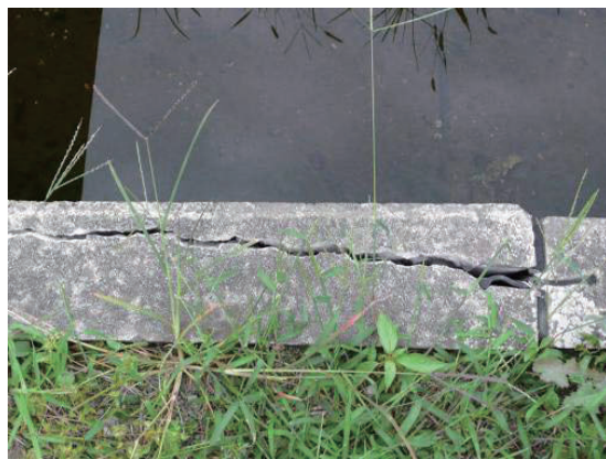
Fig.2-28 止水板から伸びるひび割れ Crack extended from the end of a water stop
