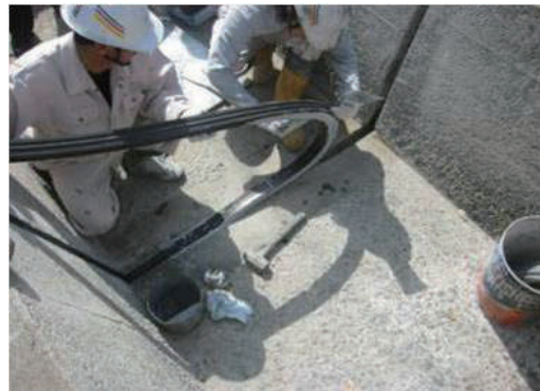
Fig.5-9 応力機能目地工法の施工状況 Construction situation of repairing joint method for concrete canal by rubber elasticity
