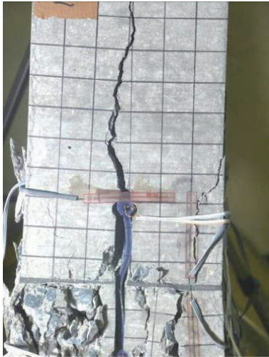
Fig.2-65 供試体2の試験後の破壊状況 Destruction situation of the test specimen2 after the loading test
