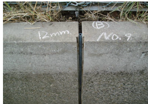
Fig.5-7 水膨張材による目地補修工法の施工状況(関東農政局, 2008) Joint repairing method by water swelling materials
