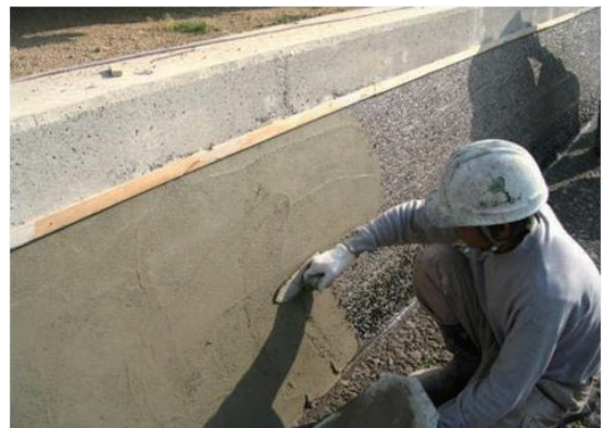
Fig.5-3 左官工法による水路表面の断面修復 Patching of irrigation canal surface by plastering method
