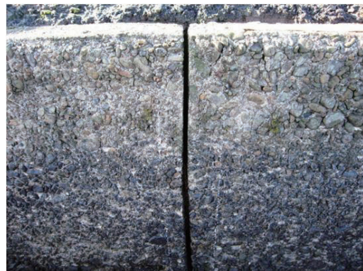
Fig.2-12 目地材の脱落 Loss of joint materials
