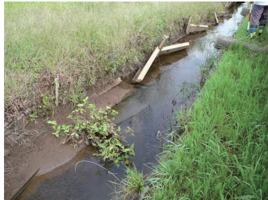
Fig.2-31 柵渠における柵板の崩落 Breakage and collapse of fence boards of a drainage canal
