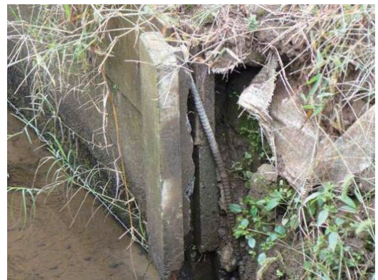
Fig.2-32 柵留め杭の破損状況 Damage to guard pile of a concrete drainage canal
