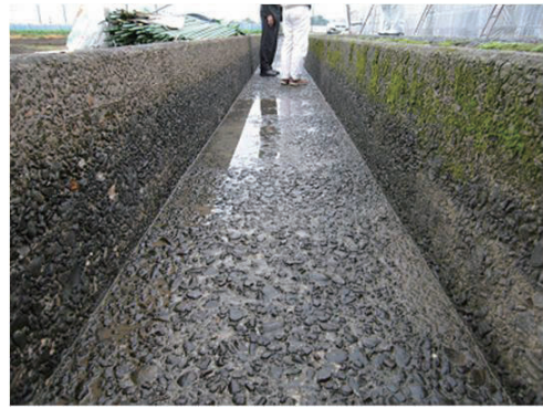
Fig.2-5 摩耗により側壁および底版コンクリートの粗骨材が露出した水路 Sidewall and base concrete of irrigation canal that coarse aggregates were exposed
