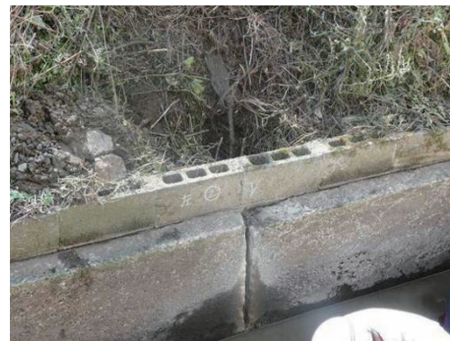
Fig.2-14 目地からの土砂の吸出しによる背面地盤の陥没 Sinking of ground at the back area of canal joint due to erosion of foundation soil
