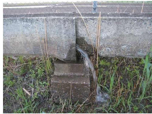
Fig.2-13 目地からの漏水 Leakage from canal joint
