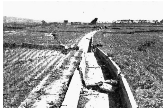
Fig.2-18 断層による躯体のずれ、目地の損傷(土木学会, 1966) Gap of concrete body and damage of canal joint due to the fault
