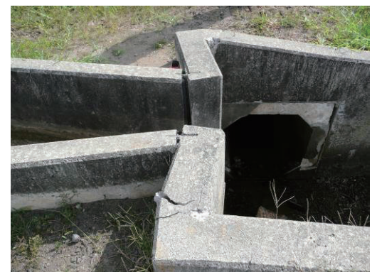
Fig.2-37 水路の突出による分水柵側壁の損傷 Damage to a diversion device by movement of the building frame
