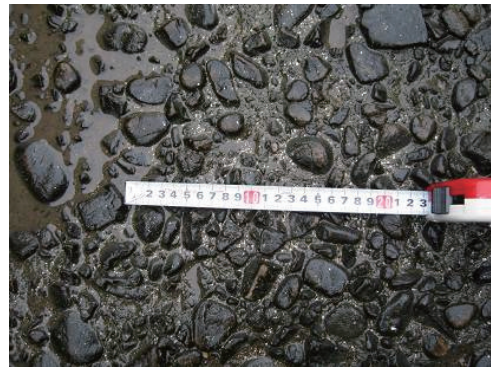
Fig.2-6 選択的摩耗による粗骨材の露出状況 Exposed coarse aggregates due to abrasion
