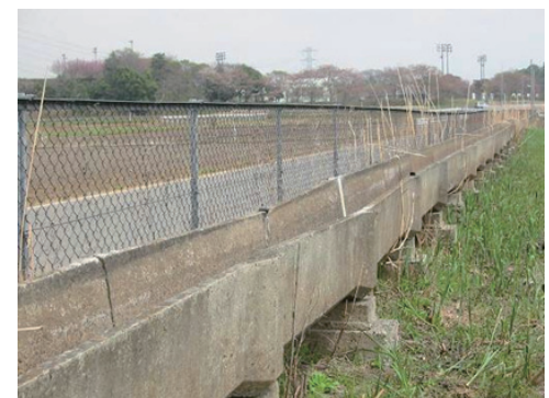
Fig.2-16 地盤沈下により不同沈下した水路 Differential settlement due to sinking of foundation
