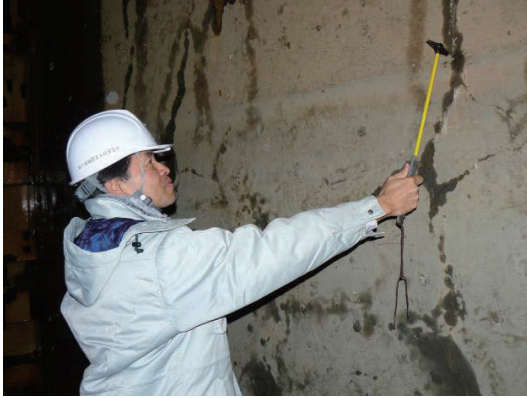
Fig.3-2 打音法による変状調査 Survey of effective events by hammer test
