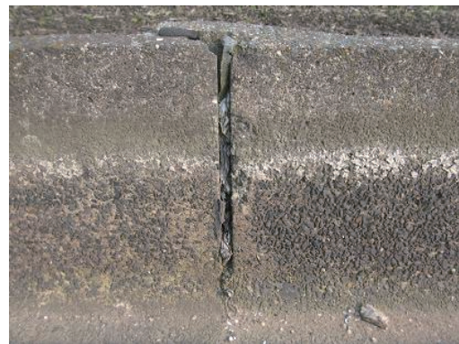
Fig.2-11 劣化した目地材 Deterioration of joint materials
