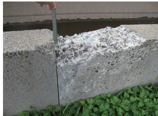
Fig.2-8 凍害による断面欠損 Losses in concrete cross-sectional area due to frost attack
