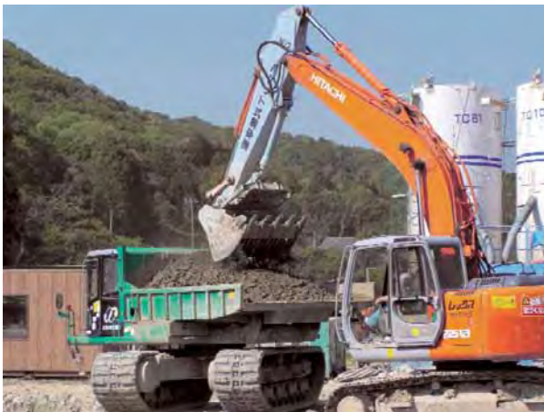
Photo.5 初期固化土の解砕・積込み状況 (バケット式解砕機) Crushing of initial-stabilized soil by bucket type crusher
