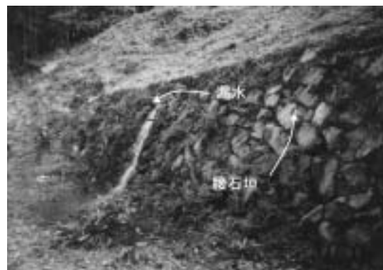
Photo 3-14 王子ため池の漏水(点d) Leakage from Ouji dam embankment (Point A)
