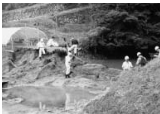
Photo 5-2 大谷ため池の決壊状況 (左岸下流側より撮影) Condition of Ootani dam breach (viewed from downstream)
