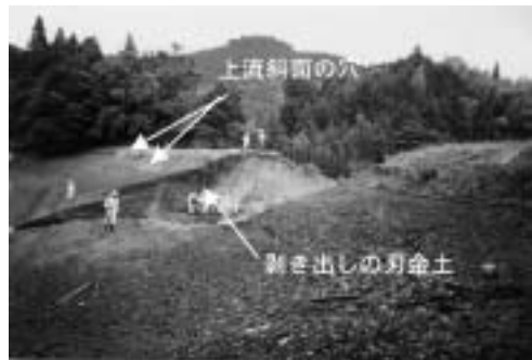
Photo 3-3 江良ため池の決壊面と上流斜面の穴 Damaged section and halls on the upstream slope of Era dam
