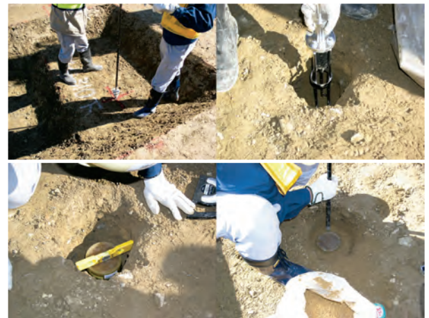
Fig.6 ワイヤレス間隙水圧計の設置状況 Views of setting up the wireless transducer
