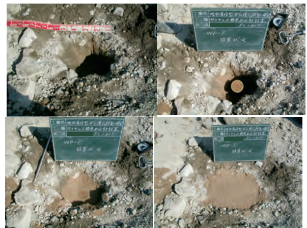
Fig.16 半透水性ゾーンにおけるワイヤレス間隙水圧計の設置状況 Views of setting up the wireless transducer in semi-permeable zone
