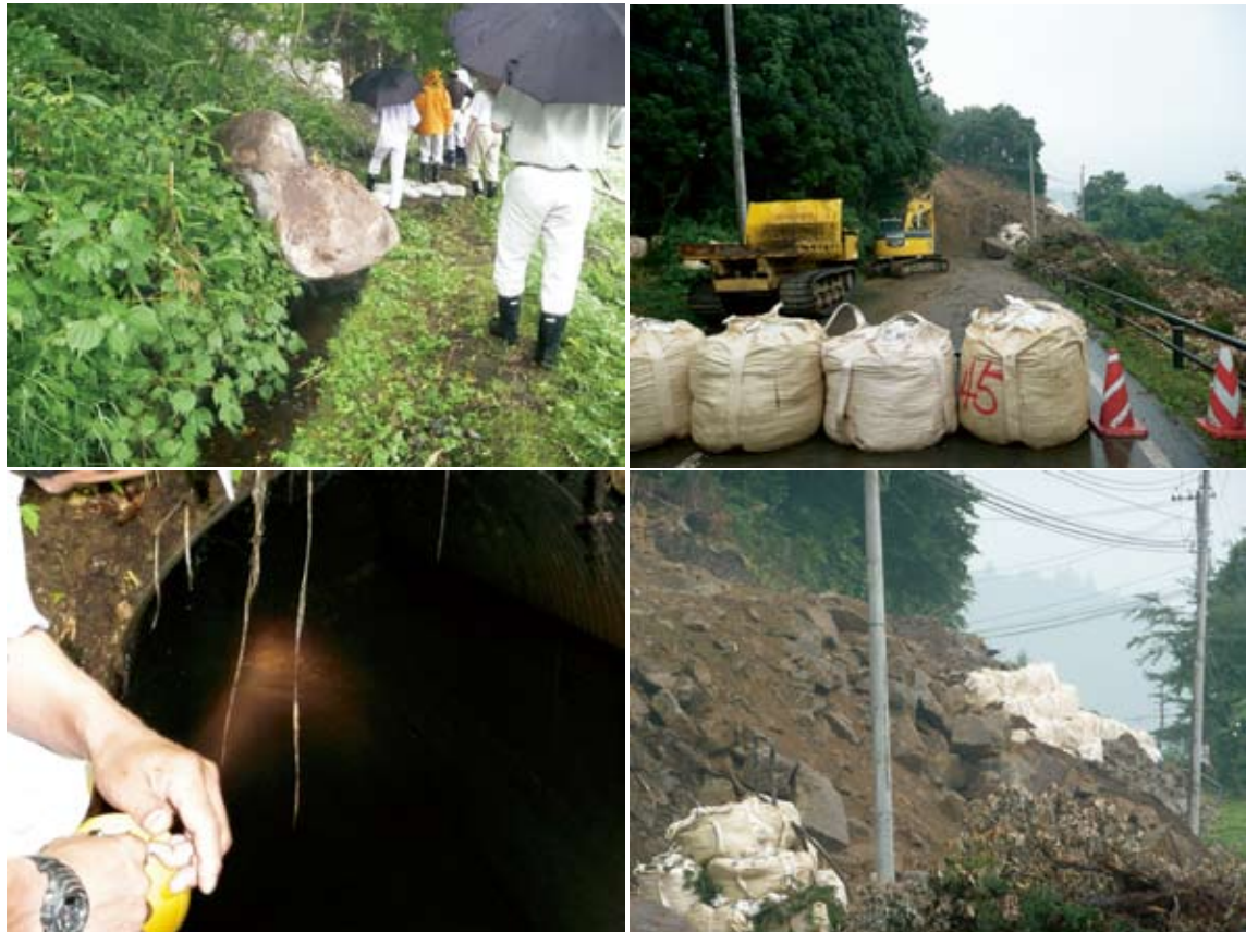
Fig.14 下真坂用水1号トンネルの被災 (左上：トンネル上流開水路への転石 (Fig.12, ①地点), 左下：トンネル出口付近の堆積土 (Fig.12, ③地点), 右：トンネル上部の斜面崩壊 (Fig.12, ②地点) Damages of Shimo-masaka channel tunnel No.1 (upper left :fallen rocks in the Shimo masaka upstream channel, lower left :deposited soil at the outlet of the tunnel, right :slope collapse over the inlet of the tunnel)
