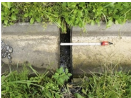
Fig.39 目地のずれ Separation of a canal joint
