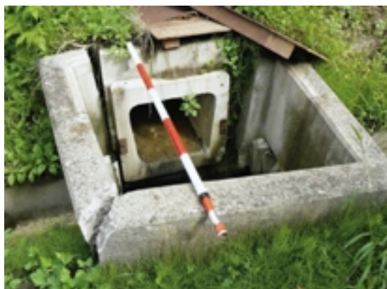
Fig.40 ボックス型水路の突出による分水柵の破損 Damage to diversion device by projection of box-type canal into the device
