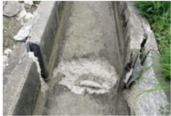
Fig.32 側壁～底版の目地部コンクリートの破損 Damage to concrete in sidewall joints and floor of a canal
