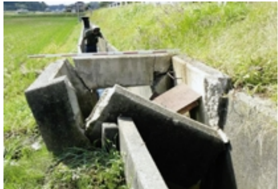
Fig.44 水路脇法面の押し出しによる分水柵の破損 Damage to a diversion device by sideways pressure from the upslope direction
