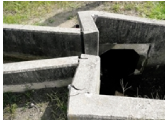
Fig.21 水路躯体の突出による分水柵の破損 Damage to a diversion device by movement of the building frame
