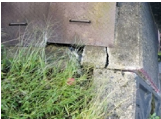
Fig.36 流入水槽に生じたひび割れ Cracking of an inflow tank
