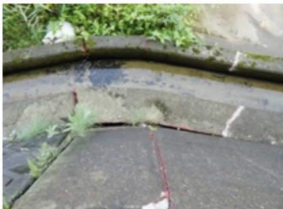
Fig.35 水路側壁に生じたひび割れとずれ Warping and cracking of a canal wall
