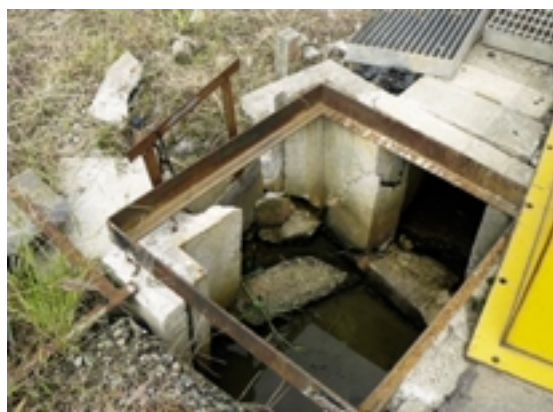
Fig.52 破損した分水枡 Damage to a diversion device
