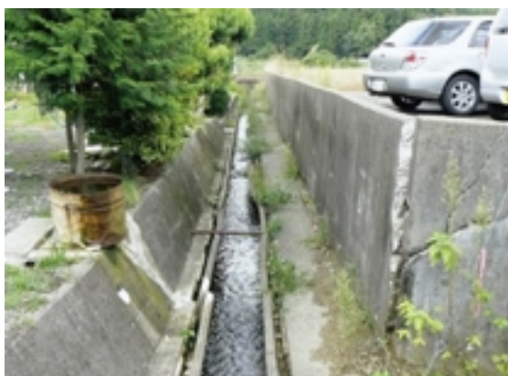
Fig.49 水路脇土留壁のひび割れや変形 Cracking and deformation of earth retaining walls beside a canal
