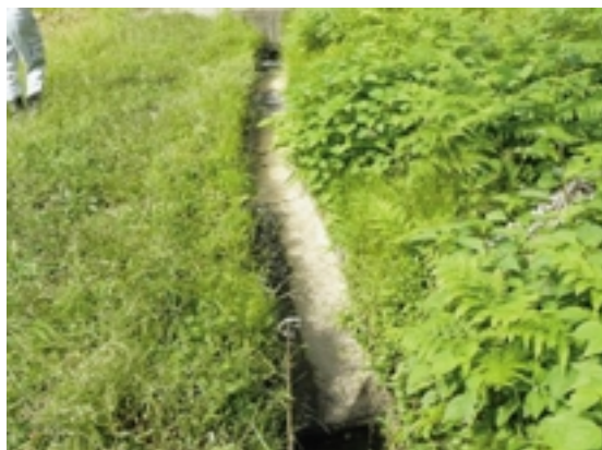
Fig.38 水路脇法面の押し出しによる水路の変形 Deformation of a canal by sideways pressure from upslope soil
