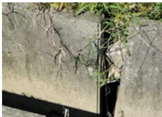
Fig.15 排水フリユームにおける目地の開き Expansion at a joint in a drainage flume
