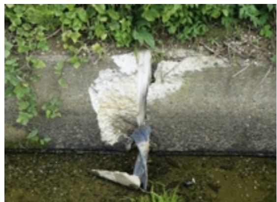
Fig.28 目地部コンクリートや止水板の剥落 Stripping of concrete and collapse of a water stop at a canal joint
