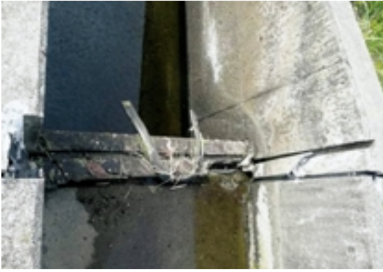
Fig.23 目地付近角落としての倒壊 Collapse of sliding timber at a canal joint
