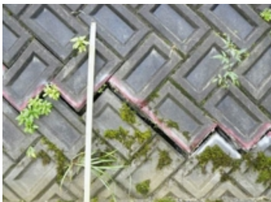
Fig.37 積ブロックの目地の開き Expansion of joints between concrete blocks
