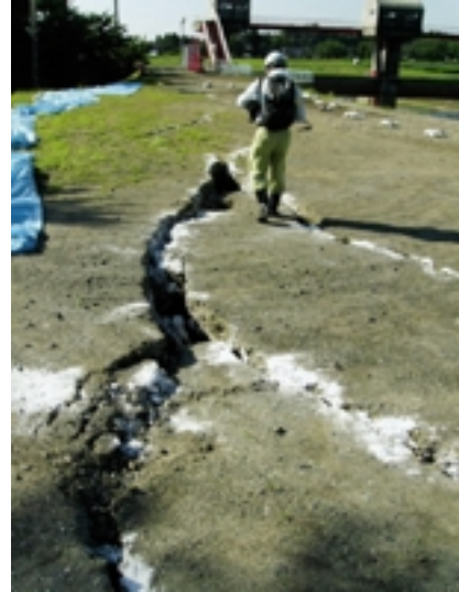
Fig.8 頭首工上流堤防天端に生じた亀裂 Cracking on an embankment at head works
