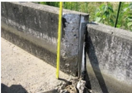
Fig.7 目地部における躯体のずれ・破損 Tilting and damage to a building frame at a canal joint
