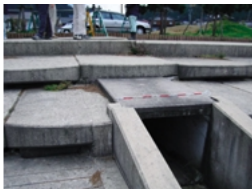
Fig.14 盛土型護岸工の変状 Damage of embankment type seawall
