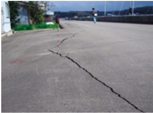
Fig.8 控え杭の突出（地盤の沈下，小牧地区） Settlement of foundation around pile
