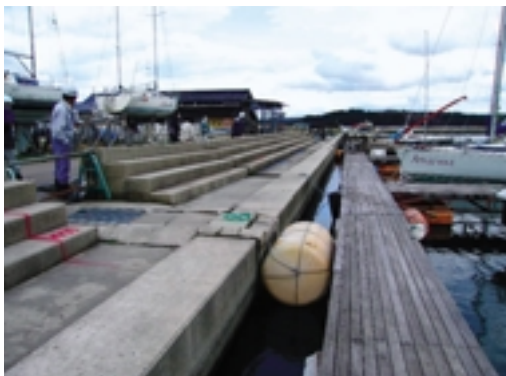
Fig.9 控え式護岸工の変状 Damage of seawall tie rod
