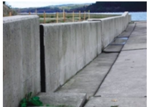
Fig.13 自立型護岸背面の変状 Damage of seawall
