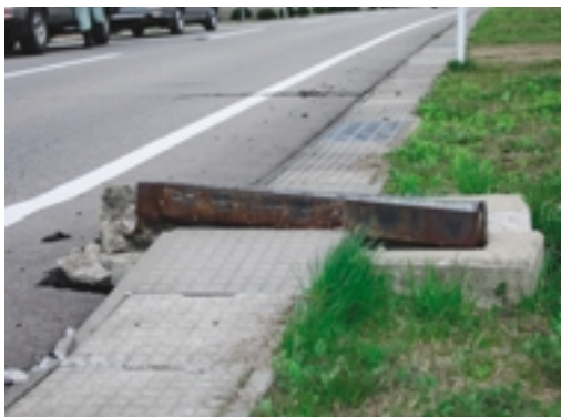
Fig.19 道路面の沈下と横断暗渠の被災 Settlement of connected road and damage to buried culvert
