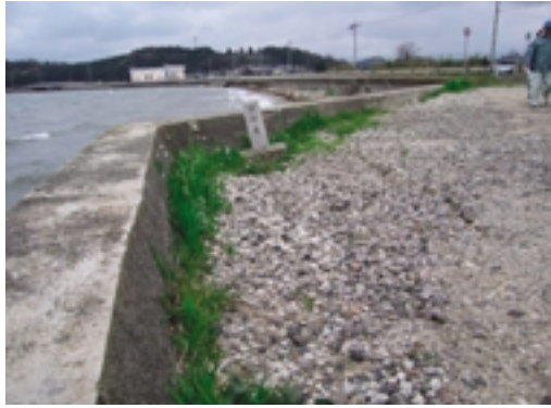
Fig.23 護岸工目地部からの背面地盤の流失 Washout of back fill sand lateral movement of seawall
