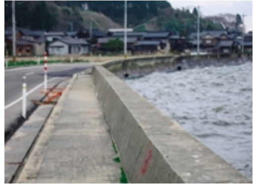
Fig.20 護岸工の移動と路面の沈下（祖浜地区） Lateral movement of seawall and settlement of road
