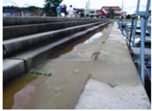
Fig.12 裏込め地盤の液状化跡 Liquefaction around seawall
