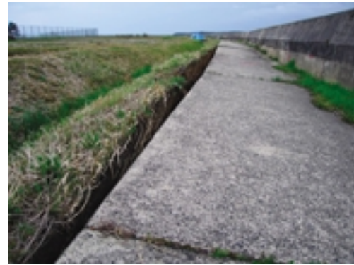
Fig.7 隣接する地盤の沈下 Settlement of backfill foundation
