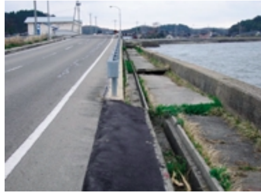
Fig.24 護岸工と道路の被災 (松百地区) Lateral movement of seawall and settlement of road
