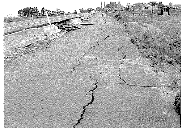
Photo 19 農道に発生したひび割れ Cracks on the farm road due to settlement
