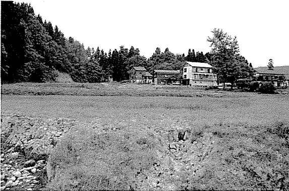
Photo 3 水田法面の崩壊 Collapse of the paddy field slope
