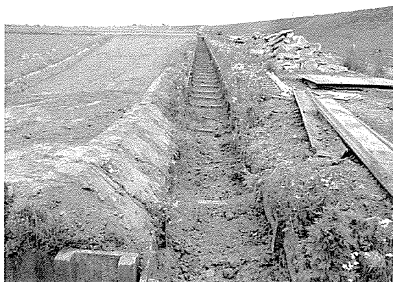
Photo 29 柵渠の埋没 Drainage canals buried by deposits
