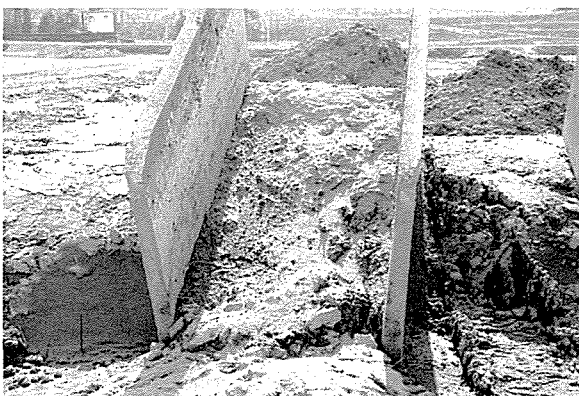
Photo 16 排水路への土砂の進入 Deposit influx into drainage canals
