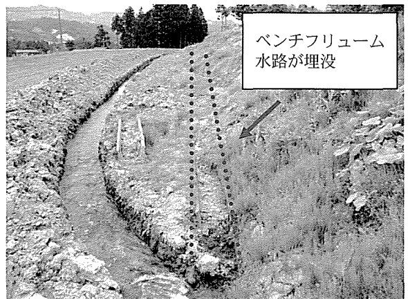
Photo 7 埋没したBF水路と水路の応急復旧 Buried bench flume canals and recovery works
