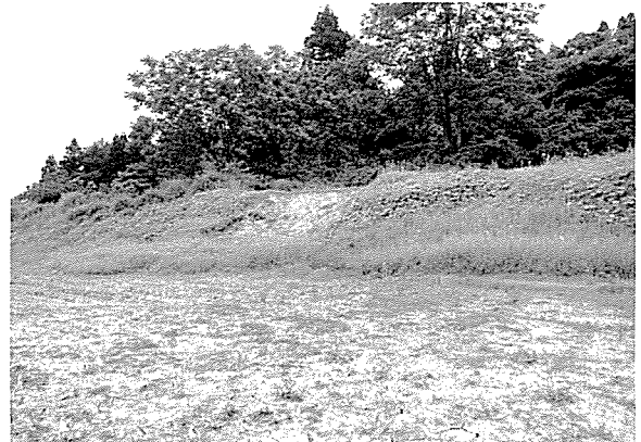
Photo 6 水田法面の崩壊 Collapse of the paddy field slope
