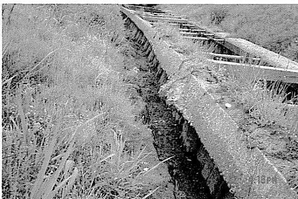
Photo 26 鋼矢板水路の損傷(深沢) Inclining of steel sheet pile canals(Fukasawa)
