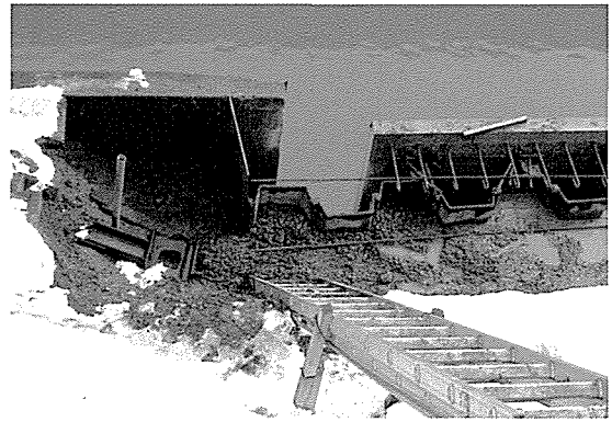
Photo 11 鋼矢板土留め工による復旧工事 Restoration works with steel sheet piles
