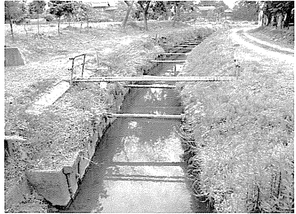
Photo 27 鋼矢板水路の損傷(花井) Inclining of steel sheet pile canals(Hanai)
