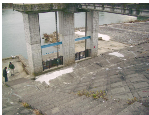
Fig.27 小千谷頭首工補修状況(04.12) A repairing situation in revetment of Ojiya Headwork
