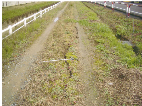
Fig.8 1号幹線水路右岸天端上の亀裂(管理用道路上)(04.10) A cracking on the maintenance road surface of right bank in No.1 main canal
