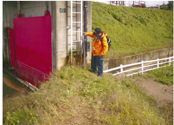
Fig.12 放流工調整ゲート門柱と地盤との段差（04.10） A difference level between a pier of a wasteway gate and ground
