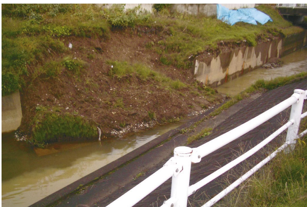
Fig.11 米沢川合流工付近の用水路側壁崩壊（04.10） Collapsing in canal left bank near a injection work of Yonezawa river
