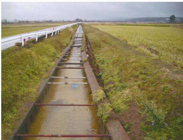
Fig.24-2 幹線排水路(鋼矢板)側部の変形(その2, 04.12) Inclining of the side wall in main drainage canal (steel sheet-pile)
