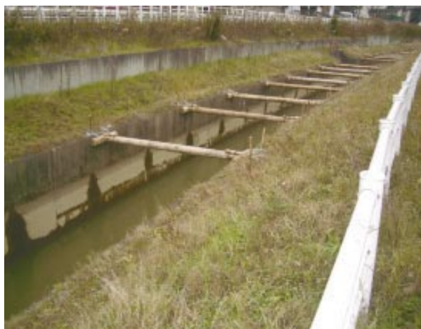
Fig.28 コンクリート水路の損傷と応急対策(04.12) Damages in the concrete retaining wall canal and emergency measures
