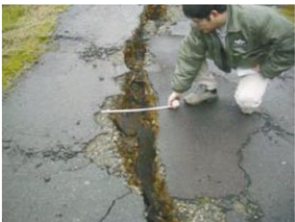
Fig.26 圃場内支線農道路面の亀裂(04.10) Cracking on the lateral farm road surface
