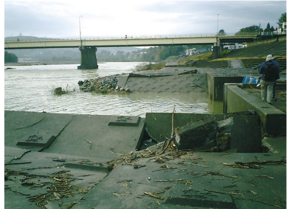
Fig.6 取水上流取入れ口護岸の損傷 (04.10) Damages of the intake revetment in Ojiya Headwork
