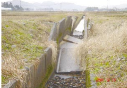
Fig.15 排水路の破損 Damage of drainage canal
