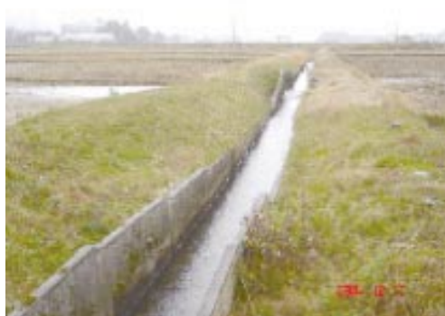
Fig.16 排水路の破損 Damage of drainage canal
