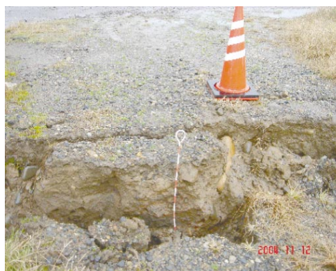
Fig.19 道路基盤の陥没 Sinking of road base
