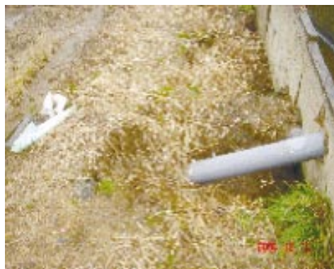
Fig.17 落水工の破損 Damage of drop
