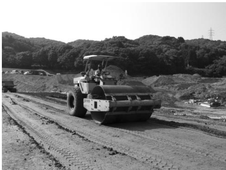
Fig.15 振動ローラによる転圧状況 Compaction of initial-stabilized soil by vibrating roller
