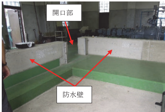
Fig. 6 防水壁 (機場内) The waterproof walls in the station
