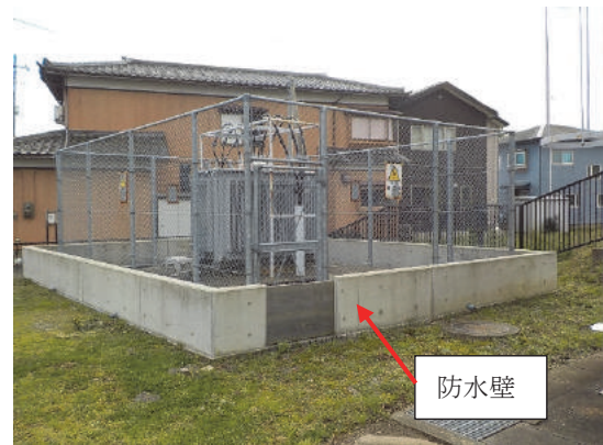
Fig. 10 防水壁 (屋外変電設備) Waterproof wall at out-door type substation
