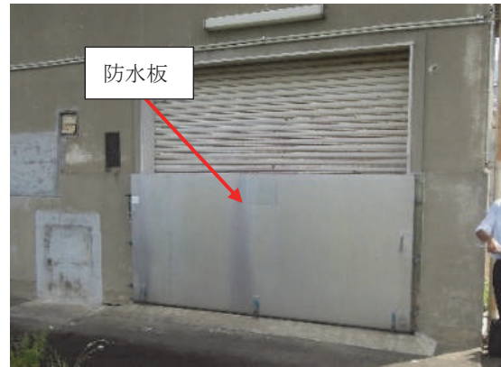
Fig. 3 防水板 (機材搬出入口) The waterproof board at the service entrance
