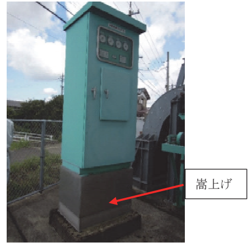
Fig. 9 嵩上げ (屋外操作盤) Raising the platform for the outdoor operation devices
