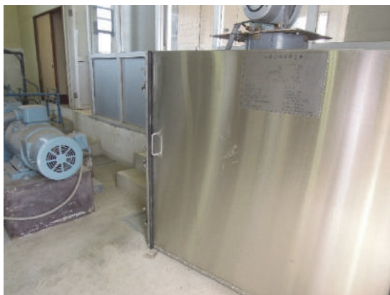
Fig. 2 防水扉 (出入口) The waterproof door at the entrance
